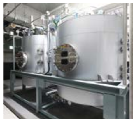
Kill tank system for wastewater treatment at Takara Bio headquarters
